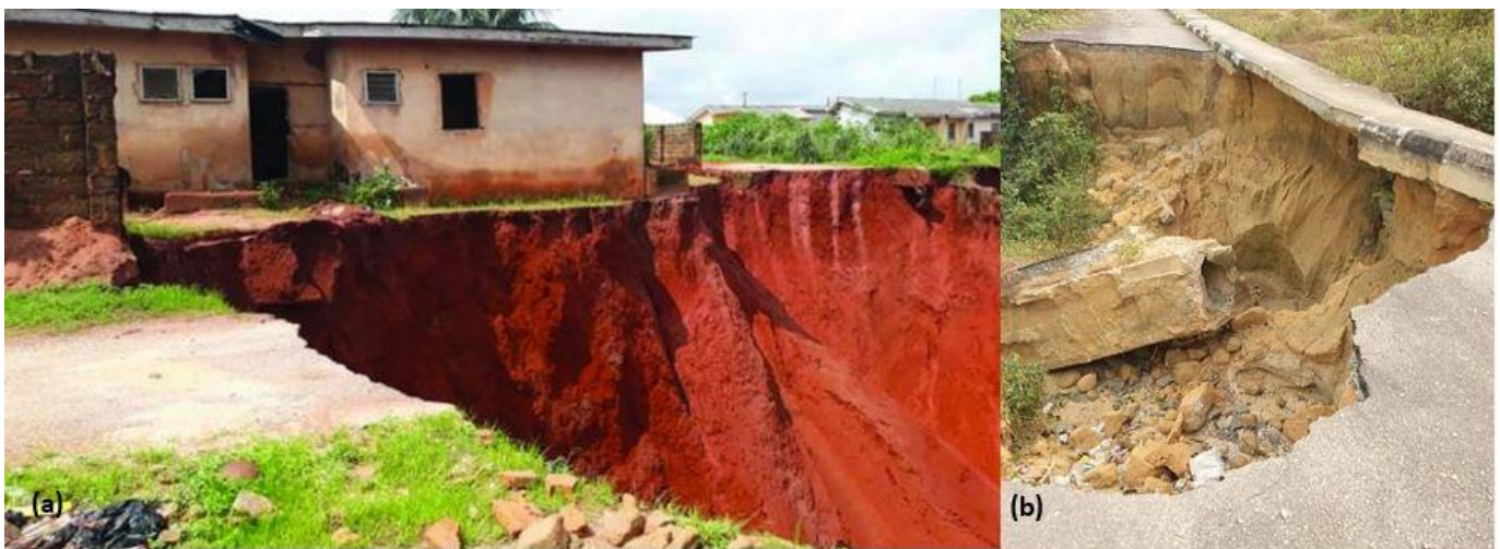
Fig. 3. (a) Residential buildings under threat by gully at Bacocco calabar, (b) Road cut by gully erosion Ikot Nkebre calabar
